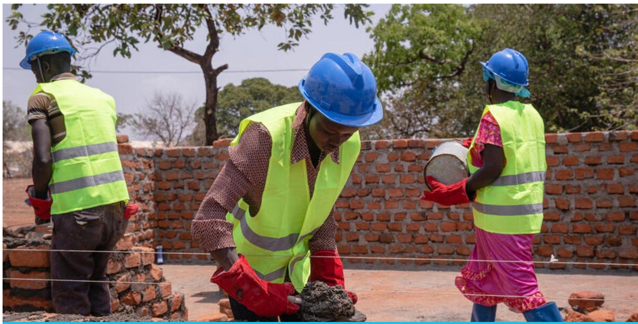
South Sudanese constructing a building in Bidi bidi Settlement, West Nile Sub-region ©UNHCR
