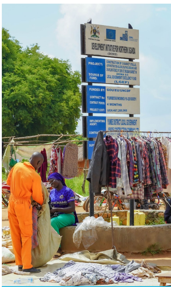
With support from EU through the DINU Programme, UNCDF is constructing modern structures for Okubani market in Bidi Bidi Refugee Settlement ©UNCDF
