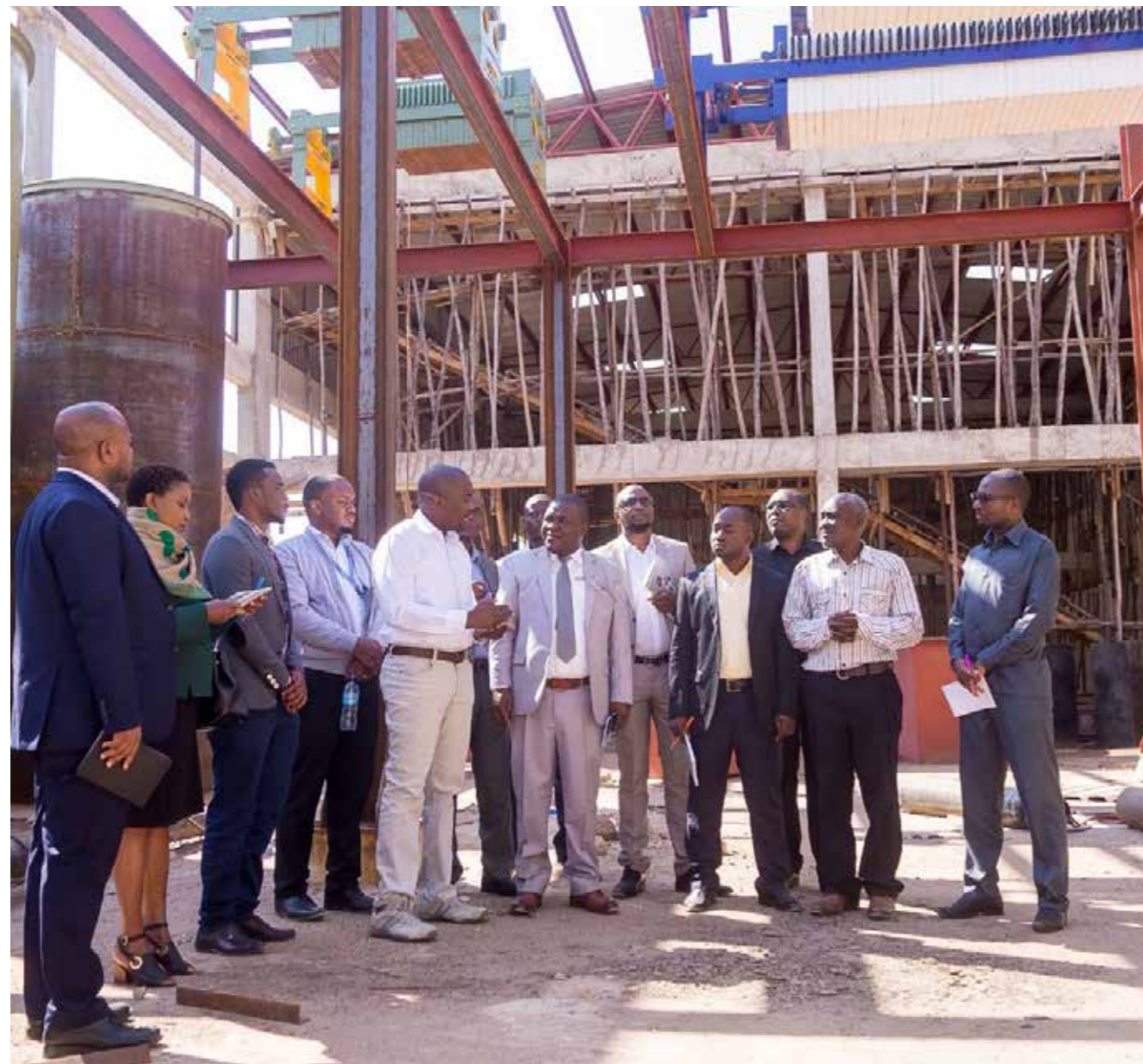
LFI Board members visiting the Mwenge sunflower processing plant during construction in Singida, Tanzania, June 2019. A Mwenge engineer is explaining implementation challenges, including equipment and civil works.
